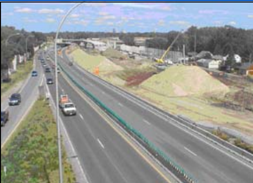
Mn/DOT wrapped up its third year of construction on the 35W / Hwy 62 project. The project should be complete in December 2010.
